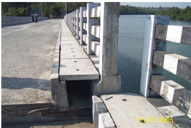
Fig. 3.12 The Ashton creek bridge in North Andaman was offset by more than a foot by extensive ground shaking
