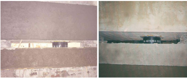
Fig. 11 The views of a two-stage system of R/C continuous beams, which separate the building from its foundation and create the seismic isolation system
