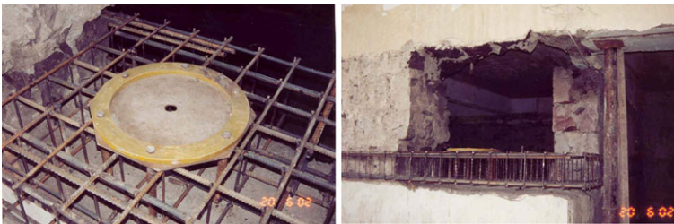
Fig. 9 The views of the lower reinforcement frames of the lower pedestal installed in the opening together with the isolator socket
