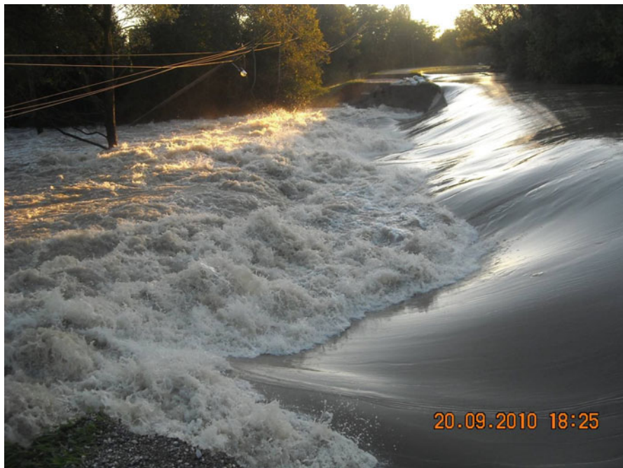
Fig. 9.3 Overflow of the right-bank Sava embankment downstream of Zagreb, 20 September 2010 ( Source: Hrvatske vode)
