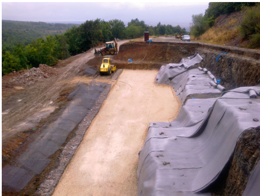
Fig. 17.7 Repairing the national road M5 between Resen and Bitola (south-western Macedonia): unloading the slided mass, stabilization with gabions, and reinforced soil surface (Photo by A. Strašeski)
