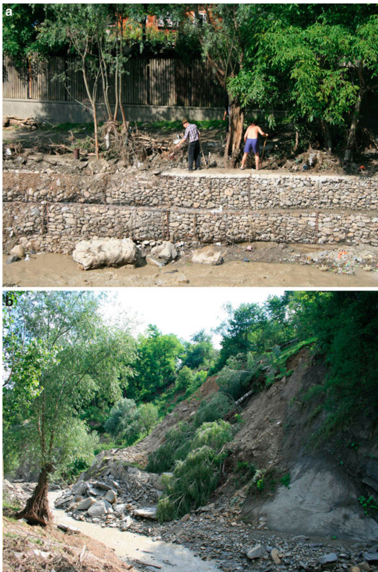
Fig. 16.5 The flash flood of July 2010 on the Drajna catchment (Cerașu, Prahova County) overpassed bank protections by 2 m (a), damaging 18 households and causing numerous riparian landslides (b) through lateral erosion (Photo by M. Micu)
