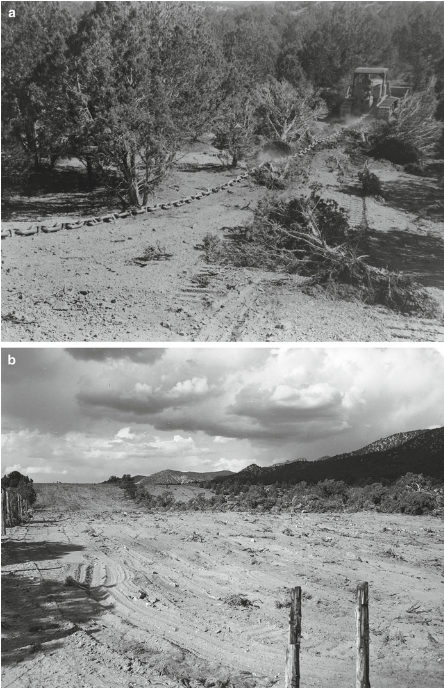
Fig. 5.13 (a, b) Removal of pinyon and juniper trees in the 1960s in Dixie National Forest in southwest Utah by chaining. (a) A large chain strung between two bulldozer tractors was dragged to uproot and topple trees. (b) After uprooted trees were removed, the area was reseeded to increase forage for livestock (Photographs courtesy of U.S. Forest Service via Special Collections, Sherratt Library, Southern Utah University)
