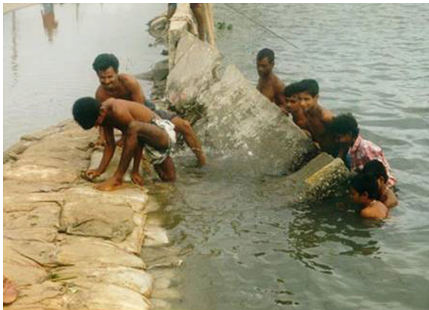
Plate 3.3 Effort of repairing a flood control structure during 1998 flood in eastern Dhaka (Source: Md. Mohiuddin Ahmed)
