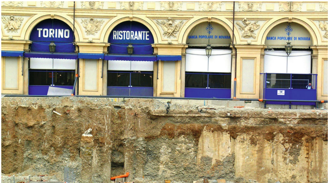
Fig. 10.1 Excavation of a soil for building a parking lot exposed a sealed soil
