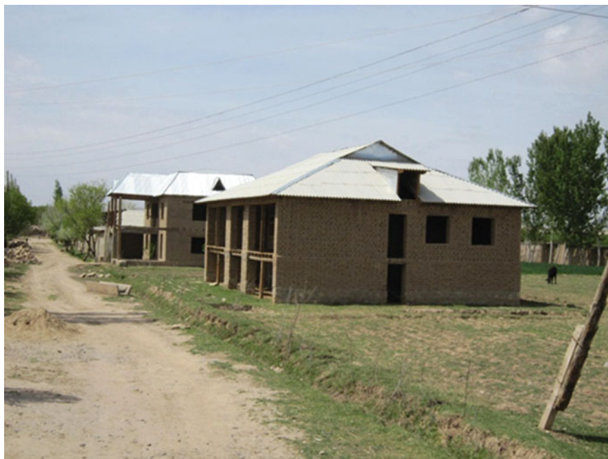
Fig. 8.11 New houses being built by returning migrants from Russia. Jamoat Saied, near Shaartuz (Photographed by Zvi Lerman, 8 April 2011)
