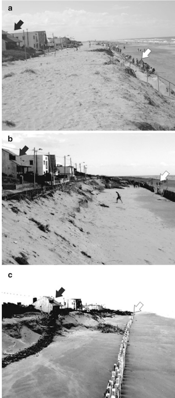
Fig. 19.13 Erosion of a rebuild foredune in Las Toninas, Buenos Aires Argentina, located on the eastern dune barrier. Photograph taken in: (a) Janeiro 2008 (b) Janeiro 2009 (c) July 2009
