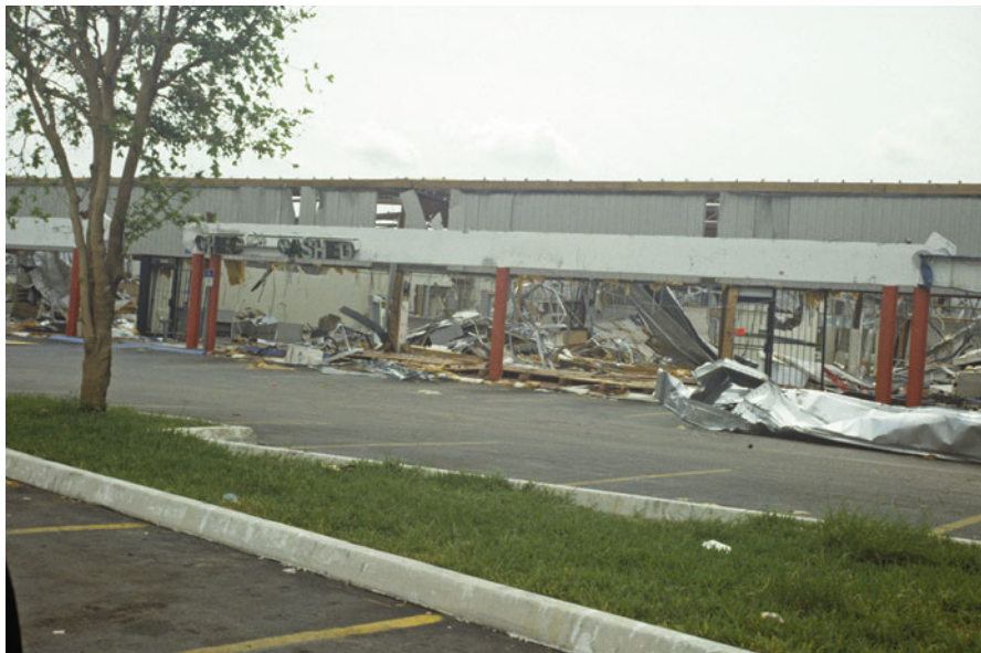
Fig. 1.4 Shopping center in Homestead, Florida, situated just south of the Miami metro area, showing complete destruction shops in this mall by Hurricane Andrew. Tornadoic winds associated with H. Andrew devastated many built-up areas, attesting to the hazards posed by hurricane-related wind fields (Photograph by C.W. Finkl)
