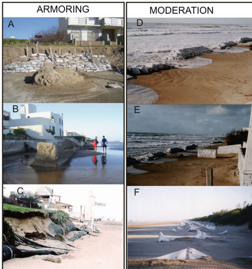
Fig. 19.17 Application of armoring and moderation classes for the dune coast of Buenos Aires. (a) Sand bags in Mar Del Tuyu for coastal protection. (b) Concrete seawalls. These rigid structure do not stop coastal retreat and collapse by undermining. (c) Geotubes. They also collapsed by wave undercutting and are very degradable with sand radiation. (d, e) Sand bags for foreshore restoration. (f) Membrane fences for backshore reconstruction
