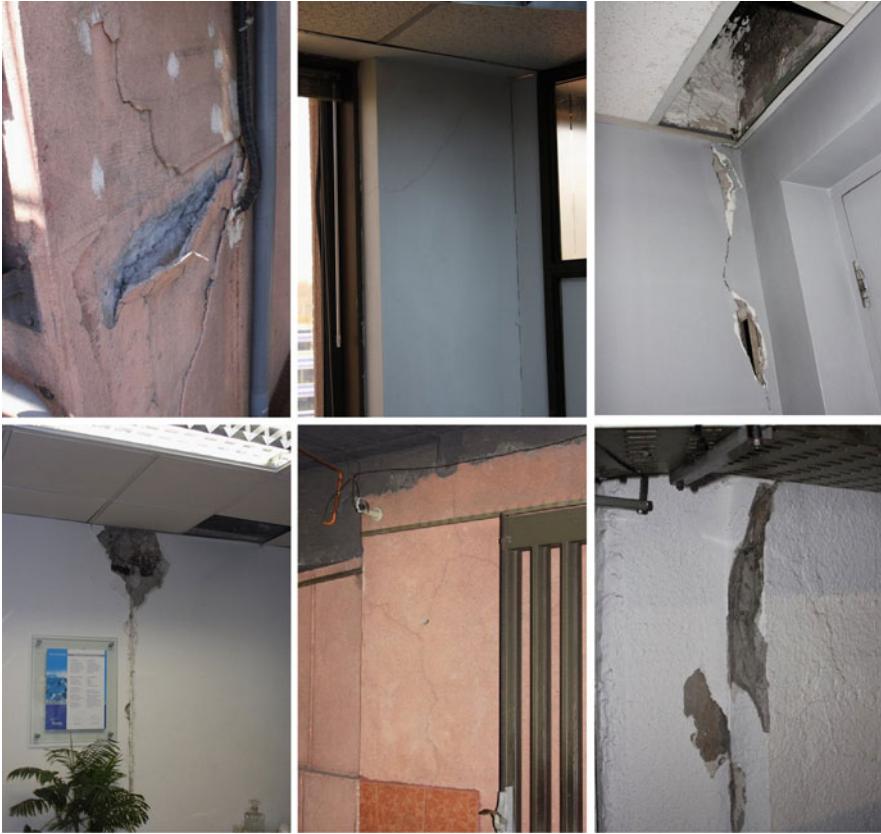
Fig. 8.16 Structural and nonstructural damage (Photo Bartolomé-Caroca)
