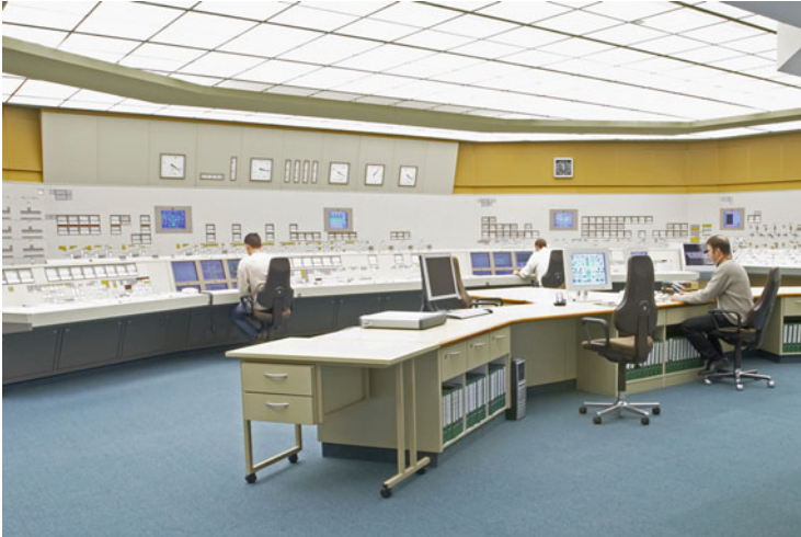
Fig. 2.1 Control room at German NPP (Photo courtesy of GfS/KSG, Essen, Germany)
