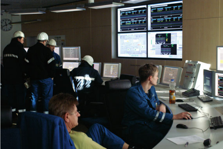
Fig. 2.7 Field operators discussing issues with the control room crew (Photo courtesy of BP Gelsenkirchen/Ruhr Oel GmbH)
