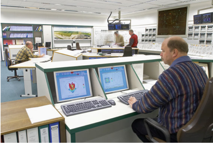
Fig. 2.2 NPP control room in Germany (Photo by GfS/KSG, Essen, Germany), because the room is windowless, the control room teams have hung up a poster with the outside view (in the back). Files with standard operating procedures on the shelves
