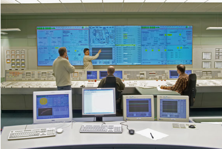
Fig. 3.14 Collaborative problem solving in an NPP control room (Photo courtesy of GfS/KSG Essen)
