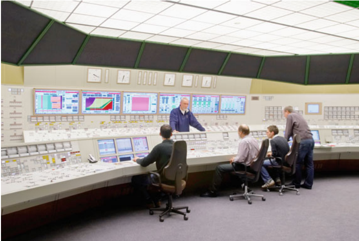
Fig. 3.12 Two operators adjusting the plant (Photo courtesy of GfS/KSG, Essen)
