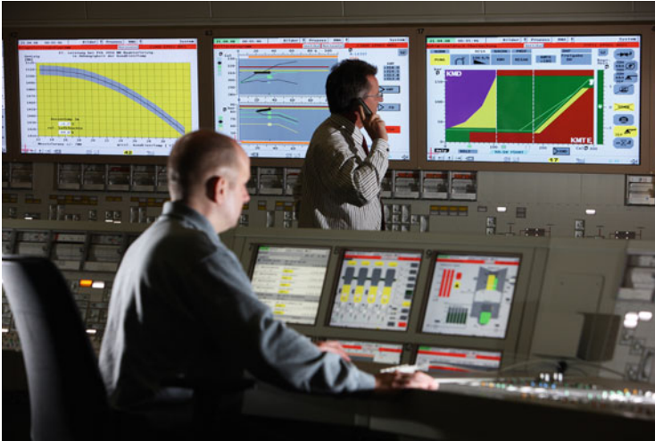
Fig. 3.11 Two control room members consulting a field operator on the telephone to clarify their observations (Photo courtesy of GfS/KSG, Essen)
