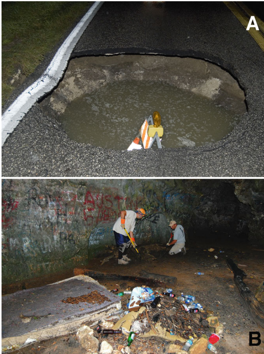
Fig. 15.14 (a) Sinkhole that opened in the middle of the road during a rain event near Tampa. (b) Extensive amounts of trash in Dames Caves in west-central Florida. The caves are often visited by locals, as they are well known to the public and have been vandalized and abused extensively over several decades. Recent efforts by the Withlacoochee State Forest, Southwest Florida Water
