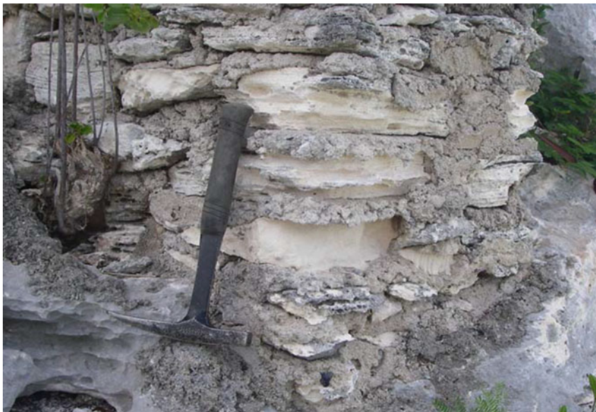
Fig. 8.23 Tafoni present in Mt. Alvernia monastery masonry work, on Cat Island. Note that the eolianite blocks weather back faster than the original mortar
