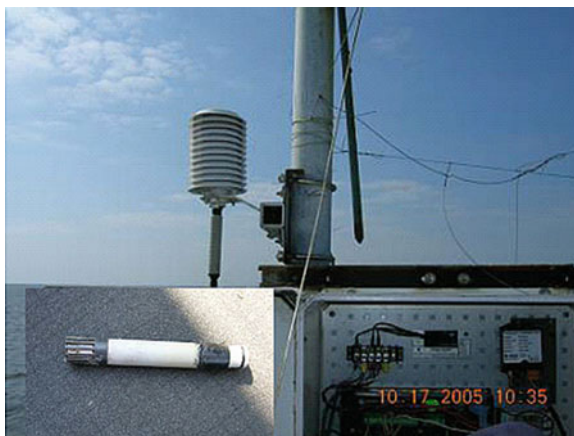
Fig. 2.2 HMP45C air temperature and relative humidity probe with data logger (Photograph provided by South Florida Water Management District)
