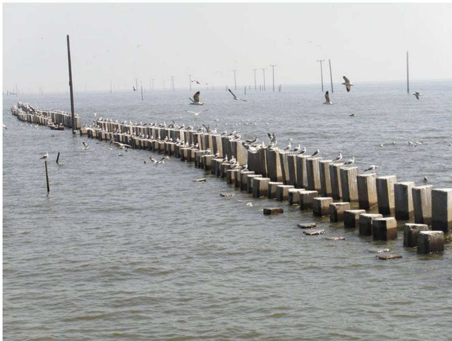
Fig. 12.2 Pilot emplacement of patented shoreline stabilization devices at Chao Phraya Delta involving wave baffles made of concrete
