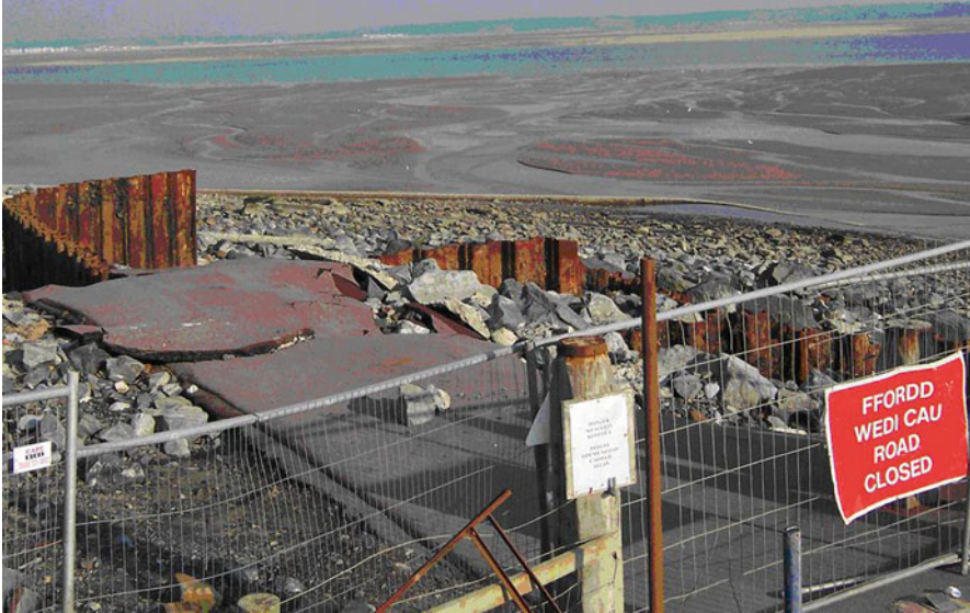
Fig. 17.11 Coastal footpath failure
