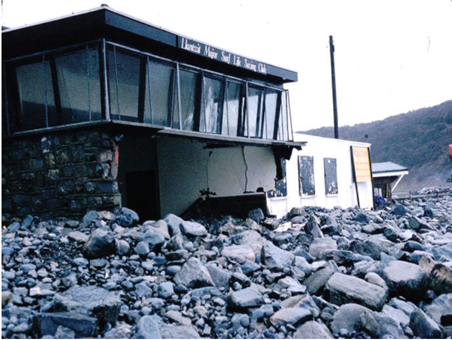
Fig. 17.2 Storm damage to Surf Life Saver Club
