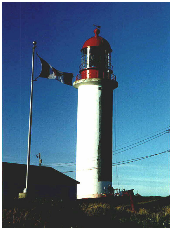
Fig. 13.4 The Cape Race lighthouse being treated with a protective, water-repellent, elastomeric coating. Courtesy of Ross Noel
