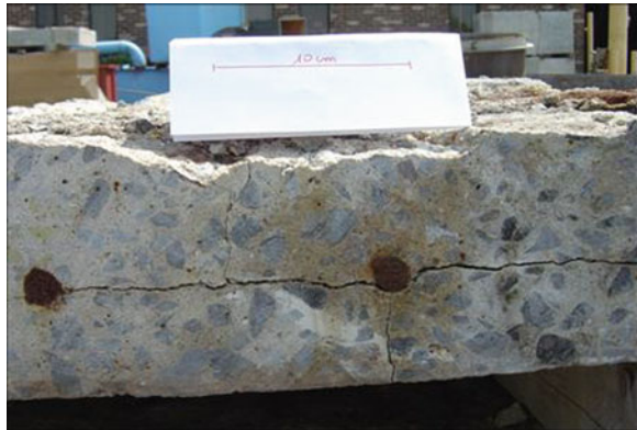
Fig. 5.3 Interface at the reinforcement level due to rebar corrosion (Naar, 2006)
