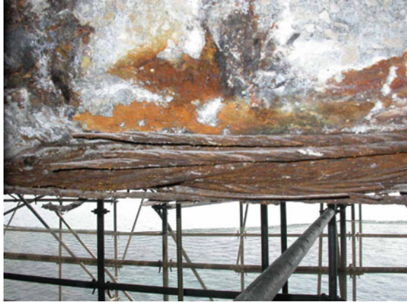
Fig. 7.2 An example of corrosion of strands with broken wires [Chauvin, 2005]
