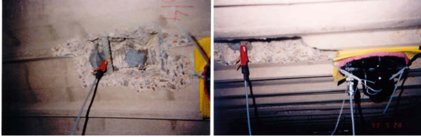
Fig. 7.17 Corrosion rate measured in-situ
