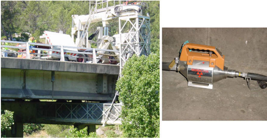
Fig. 7.5 Implementation of the technique at the intrados of a bridge deck (on the left) and a source of Iridium (on the right) – LPC France
