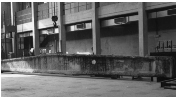
Fig. 18.6 Fire damage of pretensioned IV girder
