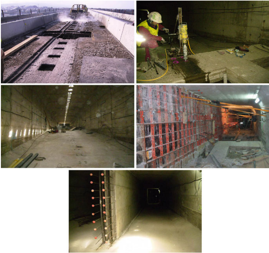
Fig. 2.16 Inner web with self-compacting concrete: drilling to place reinforcement at top slab , with hydrodemolition to avoid damage to existing reinforcement; in bottom slab , conventional drilling, accepting a certain percentage of affected bars; assembly of mild and prestressing steel
