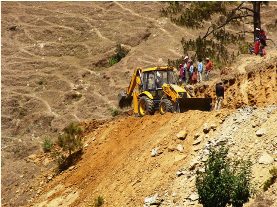
Road construction using heavy equipment in a fragile landscape (Surkhet) (Photo by PK Paudel)
