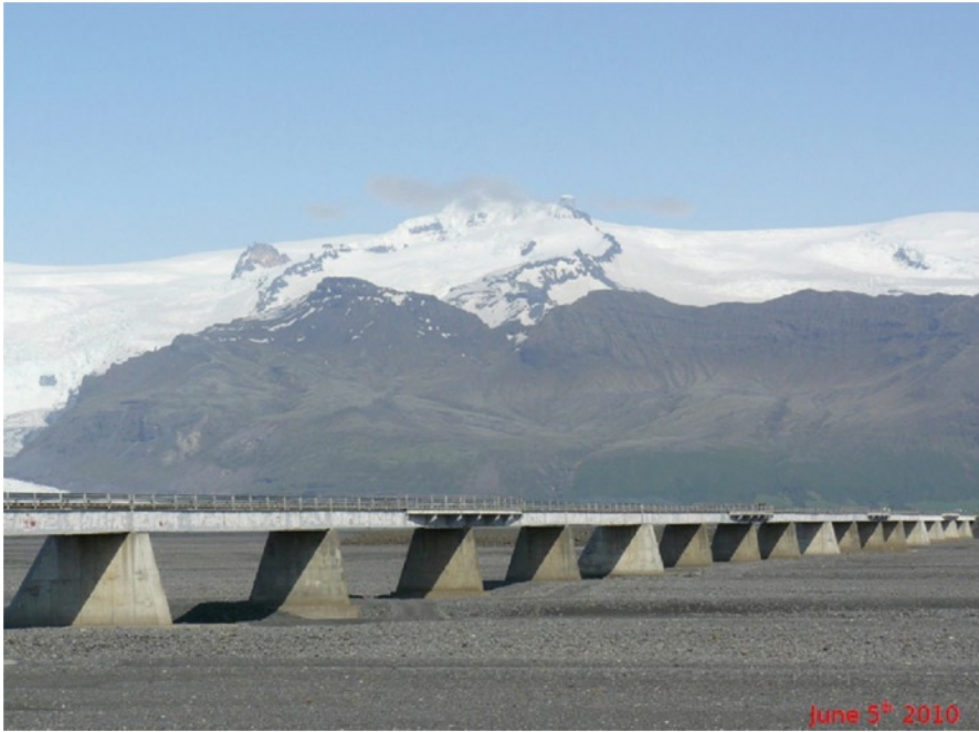
Fig. 24.4 The bridge over Skeiðará, south Iceland. The bridge was built in the early 1970s over a large glacial river. In 2009, as a result of the retreat of the Skeiðarárjökull outlet glacier, the river changed course, leaving the bridge spanning mostly dry sand
