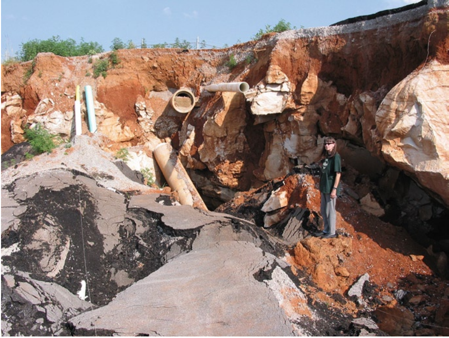
Fig. 14.2 CCKS/HERI was called to consult on the sinkhole collapse that swallowed part of a street in Bowling Green, Kentucky, USA
