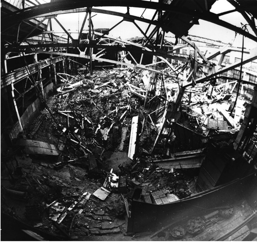
Fig. 4.6 Collapse of an industrial building in Dzerzhinsk (1992)
