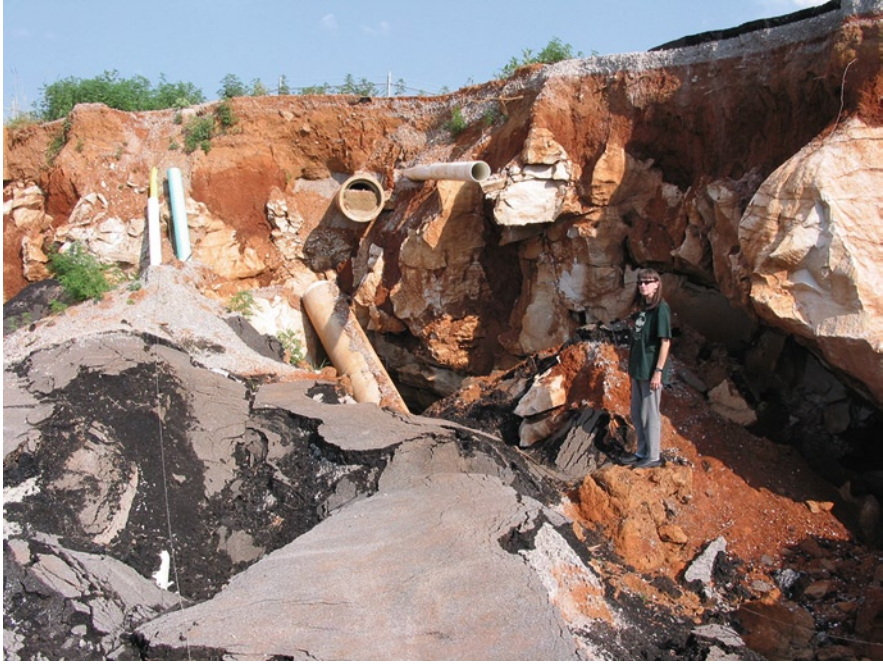
Fig. 14.2 CCKS/HERI was called to consult on the sinkhole collapse that swallowed part of a street in Bowling Green, Kentucky, USA
