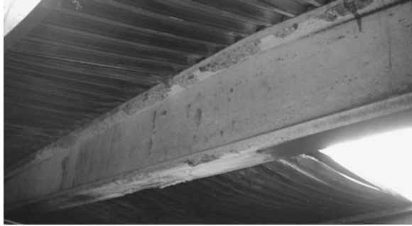
Fig. 3 Fire damage of roof girder
