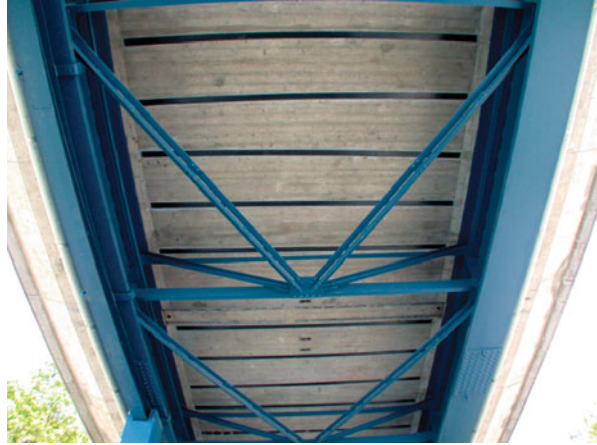
Fig. 1 View from underneath the Oberriet Bridge with the laterally post-strengthened concrete deck with CFRP strips (black)
