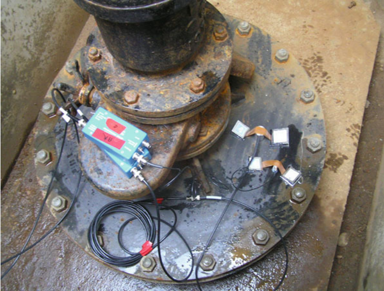
Photo 2 AE monitoring condition in service pipeline
