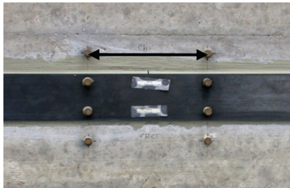
Fig. 2 Measuring points for long term strain measurement on and beside the CFRP strips. Gauge length (arrow): 200 mm
