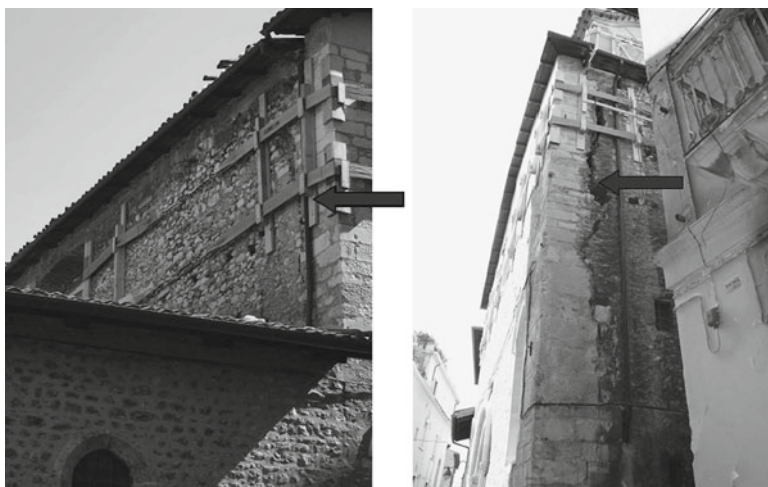
Fig. 1 Wide cracks on both sides of the façade, indicating the detachment of this last from the rest of the building
