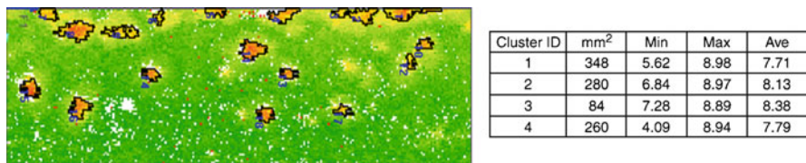
Fig. 5 Details of local corrosion and clustering results
