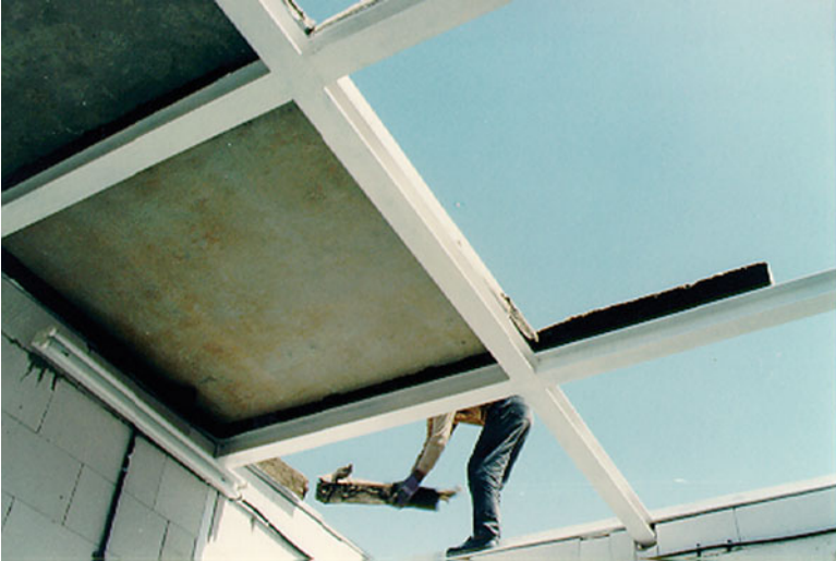
Fig. 1 Installation of the six roof slab sections on the top of the EBU
