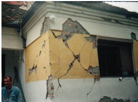
Fig. 8. Damage of two store building
