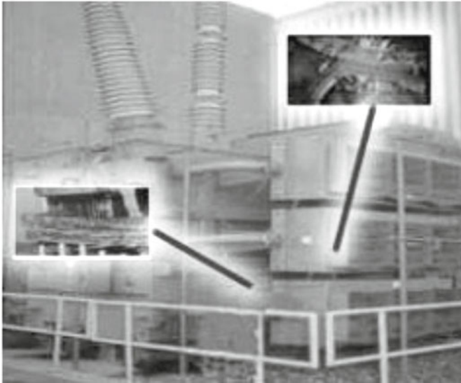
Figure 9.5. Damaged transformer ( http://www.spaceweather.gc.ca/effects_e.php ).
