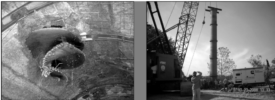
Figure 13.5. Drilling connection between well and tunnel (left), and installation of drop-shaft between the well and the tunnel (right).
