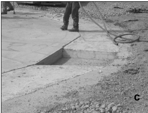
Figure 13.1. (a) Hydro-mill string on crane, (b) rebar being inserted into slurry-filled hole, and (c) final wall sections keyed into place.
