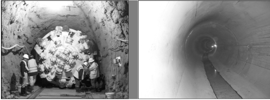
Figure 13.3. Tunnel boring machine in entrance of tunnel (left), and finished tunnel showing cast-in-place concrete liner (right).
