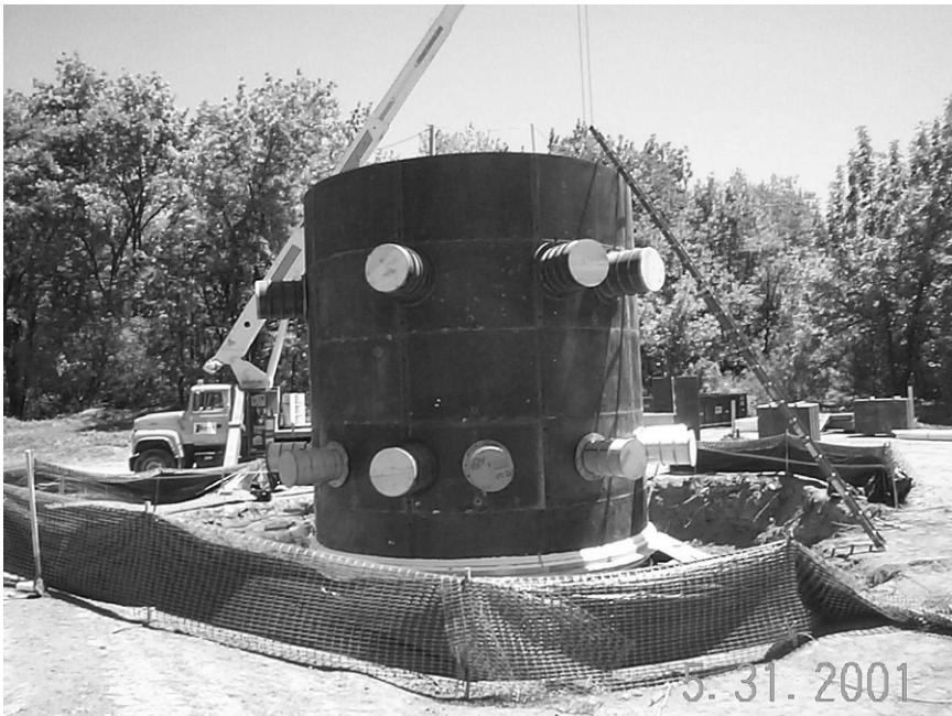
Figure 11.8. Form of the bottom section of the caisson prior to installation showing configuration of lateral portholes.
