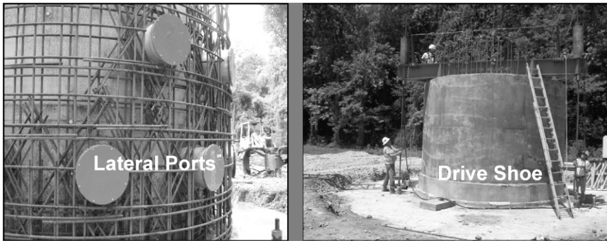
Figure 13.4. Construction of initial caisson section showing rebar and portals (left) and finished section with drive-shoe (right) ready to be “sunk.”
