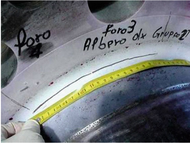
Fig. 3 Surface crack revealed by dye penetrant inspection
