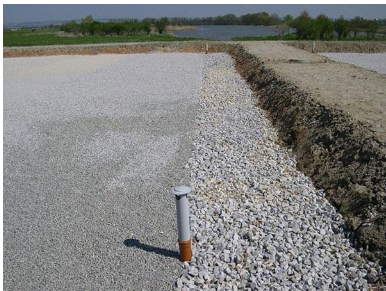
Fig. 3 Filtration bed filled with crushed rock with distribution zone filled with stones at HF CW Čejkovice, Czech Republic (Photo credit: Jan Vymazal © copyright remains with the author)
