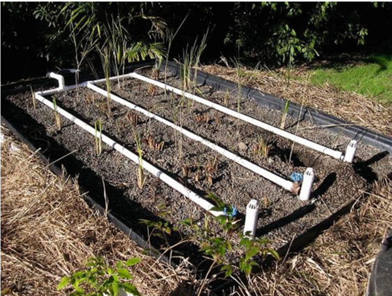
Fig. 5 On-site vertical flow CW at Bexhill, NSW, Australia, shortly after plantation (Photo credit: Jan Vymazal © copyright remains with the author)
