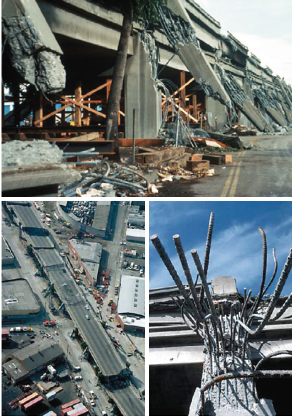
Fig. 10.8 Collapse of the Cypress Viaduct of Interstate 880 at Oakland, Loma Prieta earthquake, 1989 (photos H.G. Wilshire, USGS)
