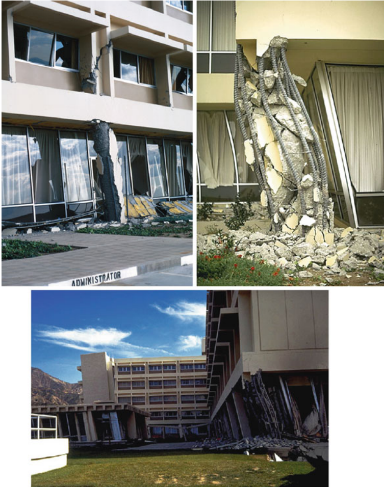
Fig. 10.6 Damage at the Olive View UCLA hospital, San Fernando earthquake (1971, photo USGS). Note the different response of columns with rectangular and spiral confinement, the shear collapse at the first floor and the relative displacement at the ground floor, estimated in 81 cm
