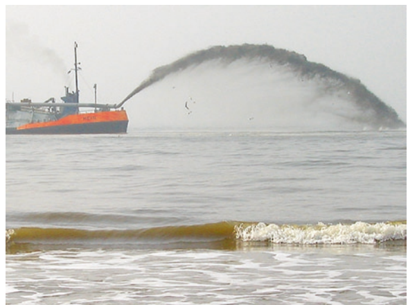
Fig. 17.5 Foreshore nourishment. Sand dredges from the bottom of the North Sea beyond the 20 m depth contour is deposited on the foreshore slope
