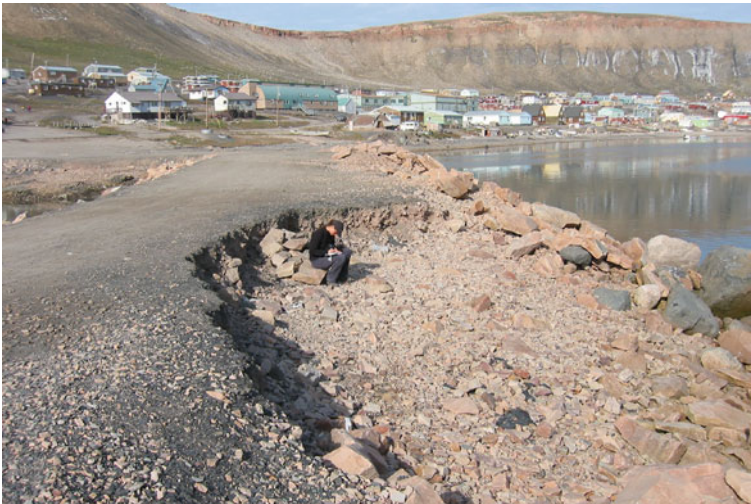
Fig. 5.2 Example of landscape hazard in Arctic Bay. Coastal erosion during an open-water, early fall storm eroded community breakwater. Photo: Trevor Bell
