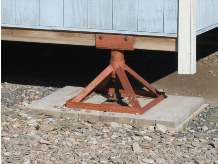
Fig. 5.3 An example of local adaptation to landscape hazard in Arctic Bay. Adjustable jack foundations mitigate the impacts of permafrost thaw and ground subsidence or heaving on buildings. Photo: Trevor Bell
