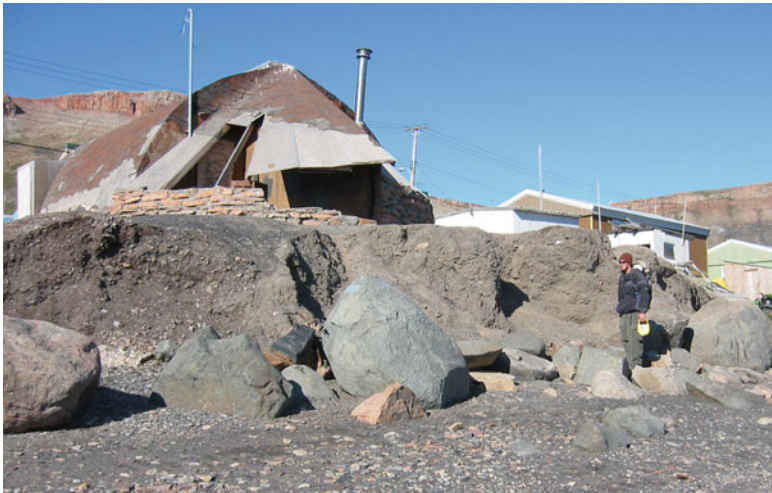
Fig. 5.4 Arctic Bay coastal armouring attempts to reduce the impact of erosion on infrastructure and land use. Protective measures were only temporary and erosion eventually undermined local infrastructure. Photo: Trevor Bell
