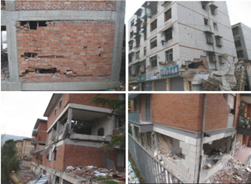
Fig. 33.1 URM infill walls damage from earthquakes in 2008 Wenchuan, China ( top ) and 2009 L'Aquila, Italy ( bottom )
