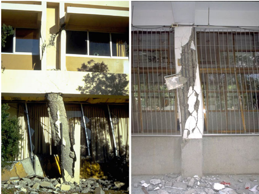
Fig. 17.1 Examples of buildings with residual displacements that lead to their demolition (Photos courtesy of NISEE, UC Berkeley)
