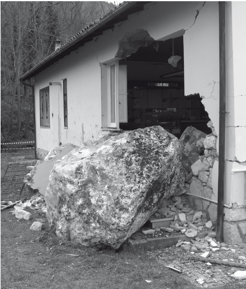
Fig. 1 Rockfall triggered by the 6 April 2009 L'Aquila earthquake near Stiffe, central Italy
