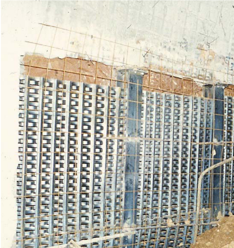
Figure 7.5 Perforated Bernold plates, placed between steel sets, act as a “skin” reinforcement.
