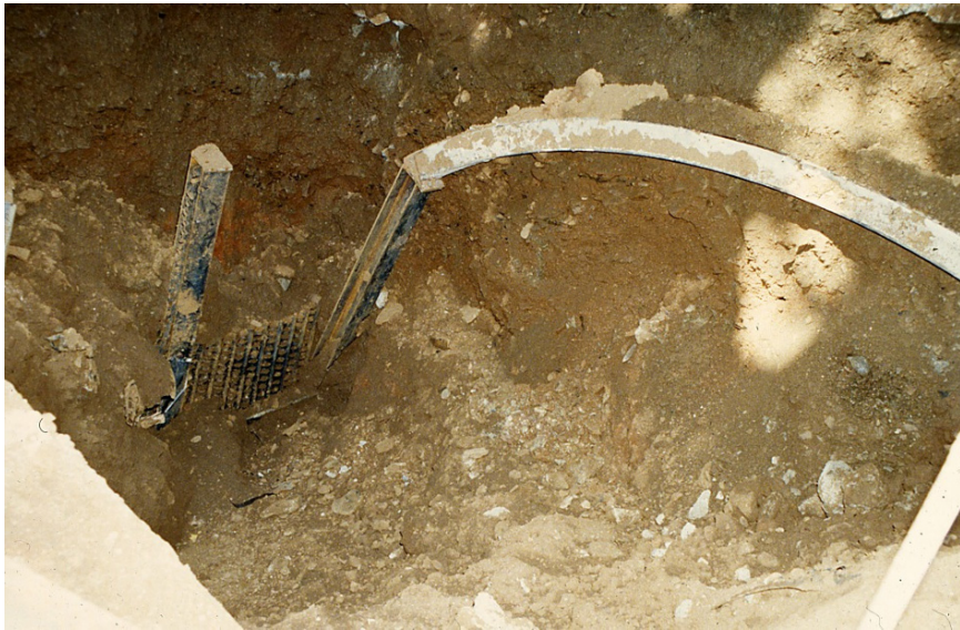
Figure 7.11 Steel sets and poles, tilted sets towards the right buttress after the failure.
