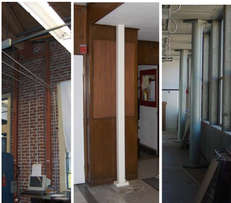
Fig. 16.3 Steel column “pre-shoring” examples from Stanford University and University of California, Berkeley (See also Plate 21 in Color Plate Section on page 468)
