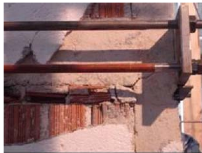
Shear cracks at beam-column joints
