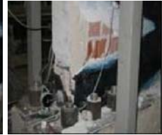
Crushing of cover concrete
