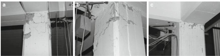
Fig. 5.4 Damaged structure after 0.2 g PGA test: (a) C3 at 2nd storey; (b) C3 at 2nd storey; (c) C4 at 2nd storey
