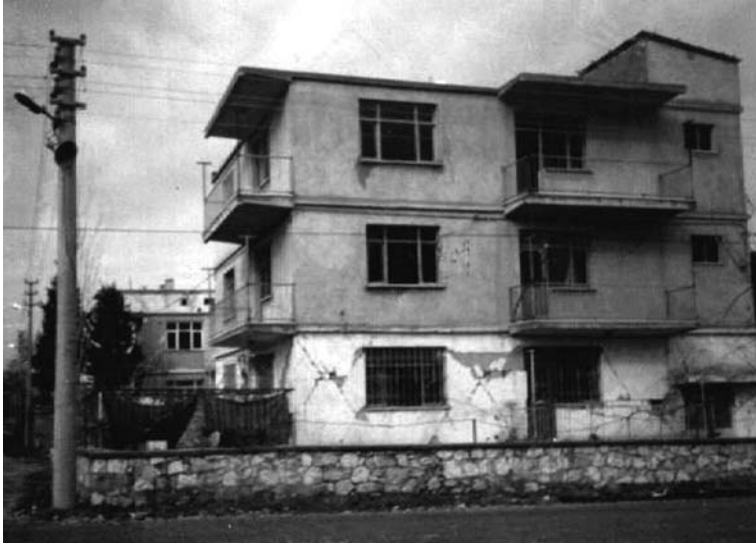
Fig. 8.2 Poor material and mortar in the ground floor (the other two stories are added later)
