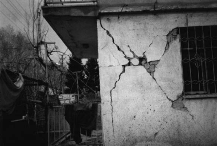
Fig. 8.4 Poor material and mortar in the wall
