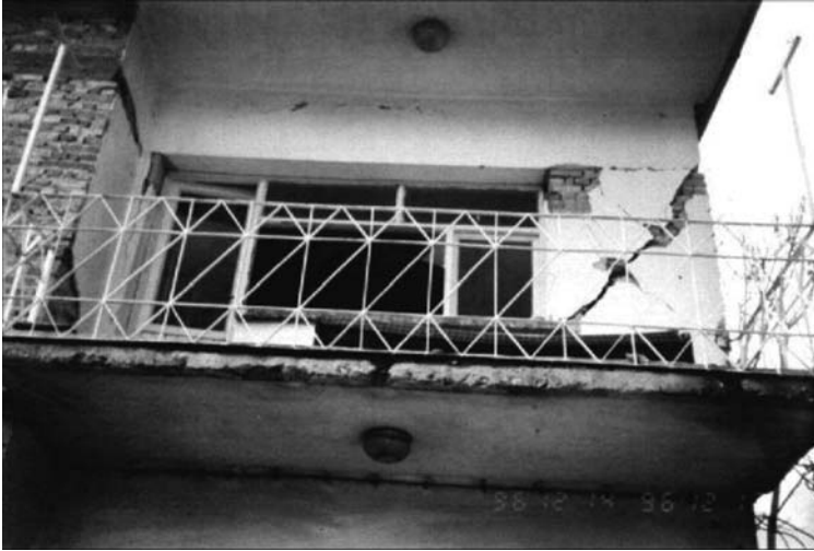
Fig. 8.12 Damage at the corner part of the wall
