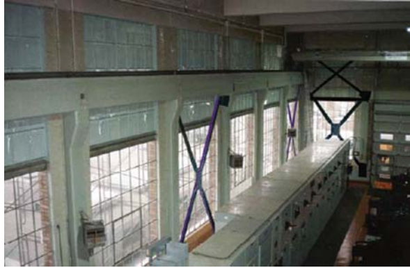
Fig. 6.13 Friction dampers in Pump House Building
