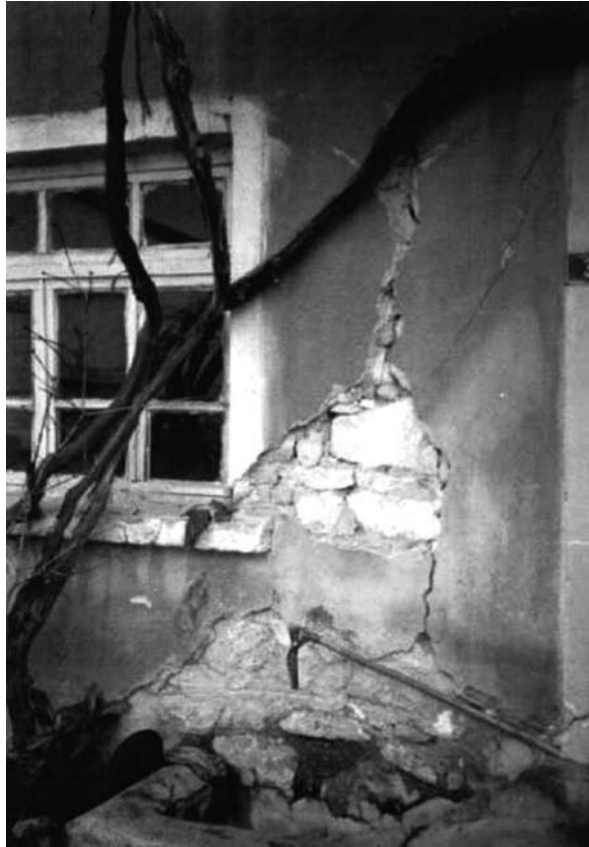
Fig. 8.1 Poor material and mortar in the wall
