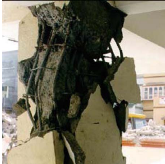
Fig. 6.2 Shear failure of column (See also Plate 5 in Color Plate Section on page 457)
