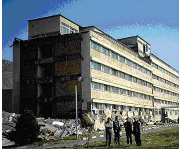
Fig. 16.1 Story collapse vertically downward without significant lateral movement (note vertical alignment with adjacent uncollapsed wing) (See also Plate 19 in Color Plate Section on page 467)
