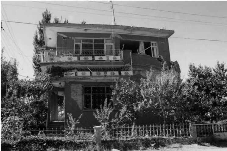
Fig. 8.13 Large openings in the walls
