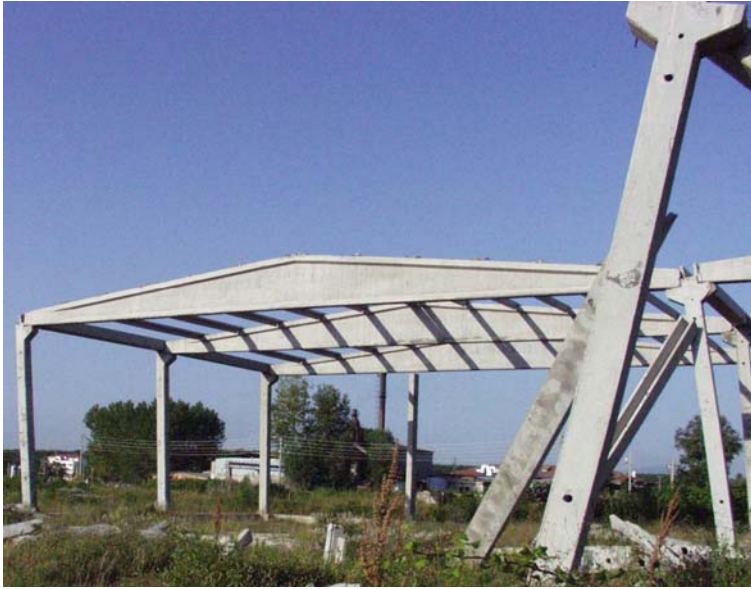
Fig. 9.1 Collapsed precast industrial building near Adapazarı following the 1999 Kocaeli Earthquake
