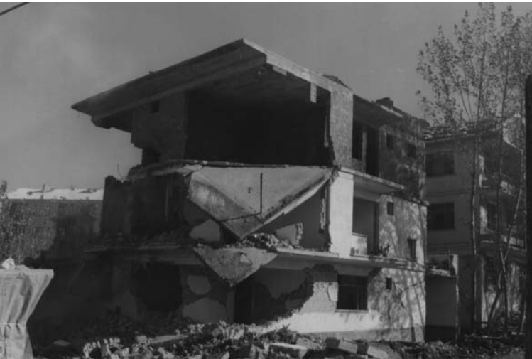
Fig. 8.5 Substandard wall units
