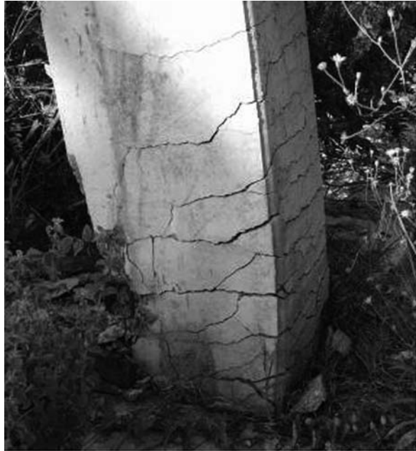
Fig. 9.3 Flexural hinge at base of cantilevered, precast column
