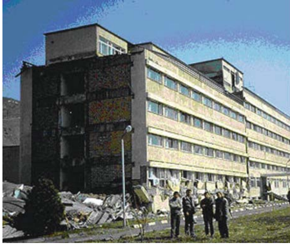
Plate 19 Story collapse vertically downward without significant lateral movement (note vertical alignment with adjacent uncollapsed wing) (see also Fig. 16.1 on page 330)
