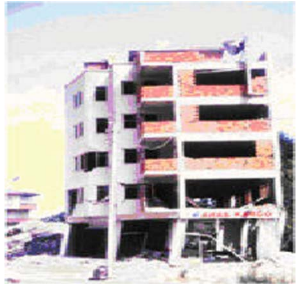
Fig. 16.2 Side sway mechanism with incipient collapse (See also Plate 20 in Color Plate Section on page 467)
