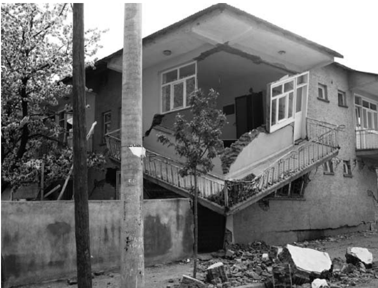
Fig. 8.11 Lack of integrity between walls
