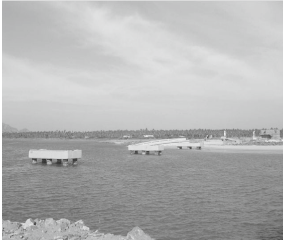
Fig. 6 All spans of the Melamanakudi Bridge came off their bearings. The end spans drifted upstream, while the middle spans sank into the river (Photo: Sheth et al., 2006).
