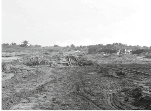
Fig. 7 Damaged railway line between Nagore and Nagapattinam in Tamil Nadu (Photo: Sheth et al., 2006).
