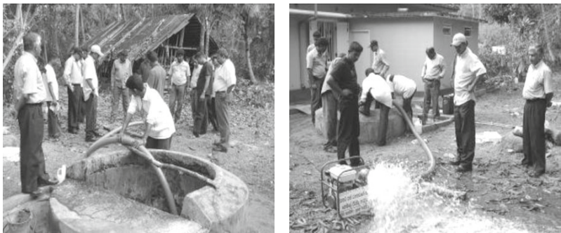
Fig. 3 Cleaning a typical drinking water well after the 2004 Tsunami in Sri Lanka (Courtesy: Jannick M Christensen).
