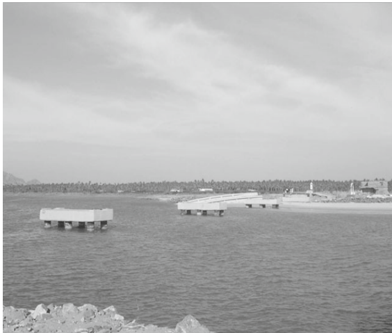
Fig. 6 All spans of the Melamanakudi Bridge came off their bearings. The end spans drifted upstream, while the middle spans sank into the river (Photo: Sheth et al., 2006).
