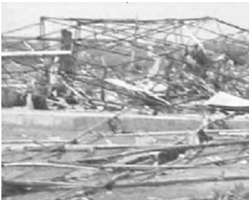
Production Godown Blown Off
