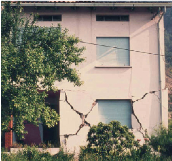
Figure 6. Diagonal crack in masonry walls and loss of corner wall URM masonry' R.C. floors (EMS)
