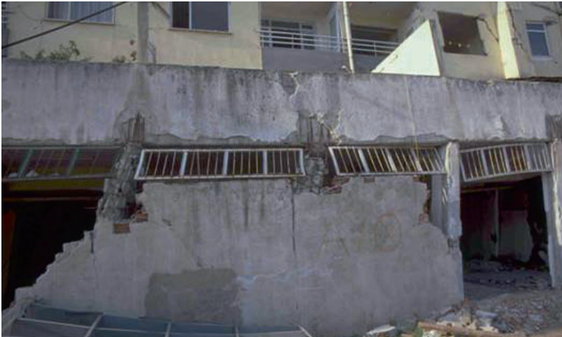
Figure 11. Damages on the R.C. frame structure due to masonry infill (SGEB, 2004)
