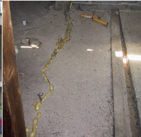
Figure 8. Damages on the top (fifth) slab
