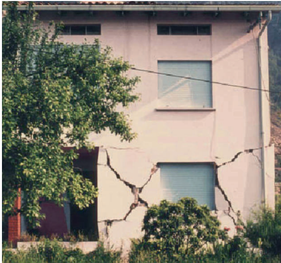
Figure 6. Diagonal crack in masonry walls and loss of corner wall URM masonry' R.C. floors (EMS)
