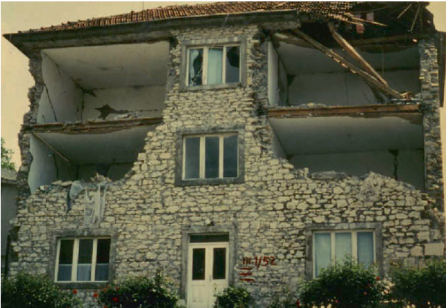
Figure 7. Stone masonry building with wooden floors, earthquake in Montenegro 1979 (EMS)
