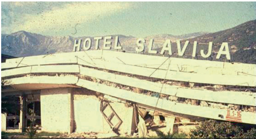
Figure 8. Soft-story and non-symmetrical structure Montenegro 1979
