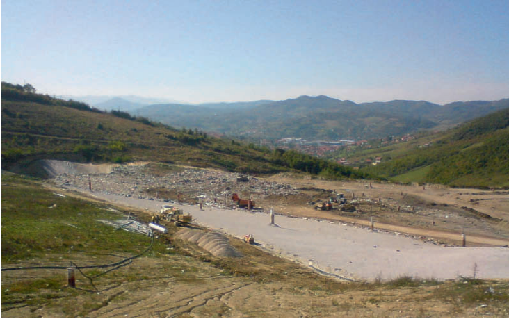
Figure 12. “Smiljevici” – sanitary landfill in Sarajevo, B&H (Serdarevic, 2007)
