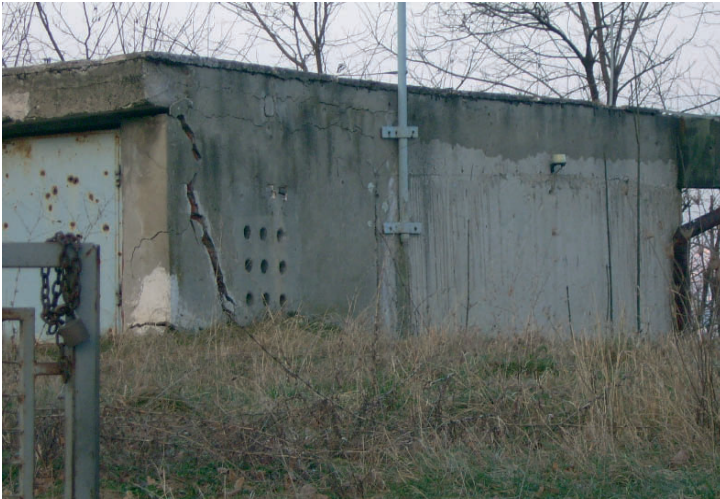
Figure 17. Damages of water tank “Hambina Carina” – upper side
