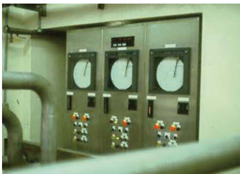
Figure 8.4 Temperature control panel
