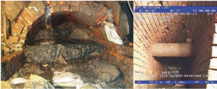
Fig. 13.4 Unattended collapses and intrusions of other services
