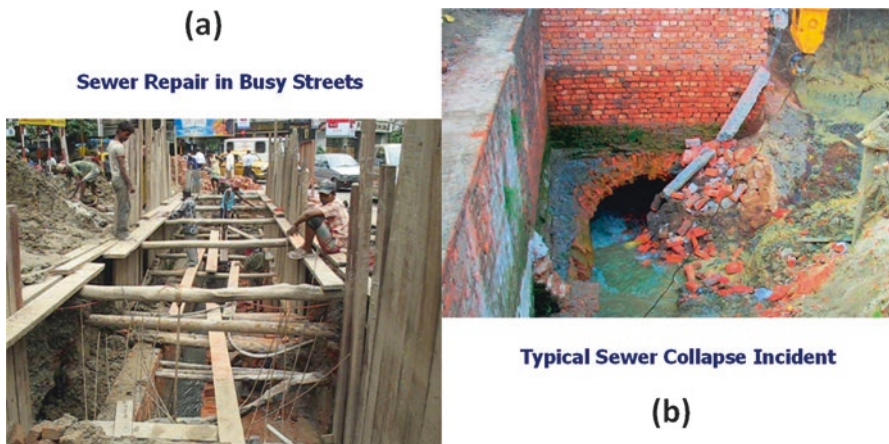
Fig. 13.5 (a) Sewer repair work on a busy street in Kolkata. (b) Typical sewer collapse incident
