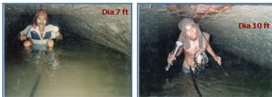
Fig. 13.3 Silted up unattended sewers down underground
