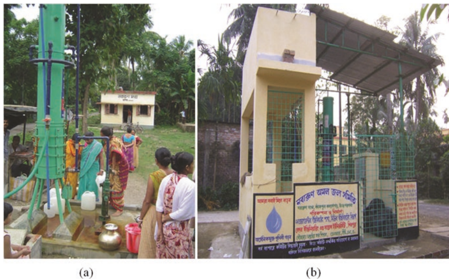
Fig. 10.7 (a) The photograph of the arsenic removal unit at Nabarun Sangha, North 24 Parganas, in 2005 shortly after installation and (b) photograph of the same unit in 2009 following continuous upgradation by the village water committee
