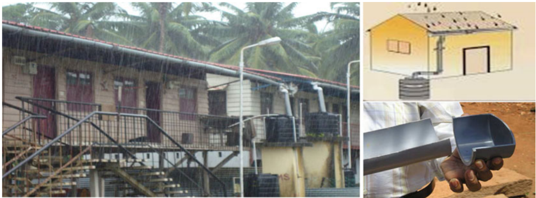
Fig. 8 Rooftop rainwater harvesting in group houses
