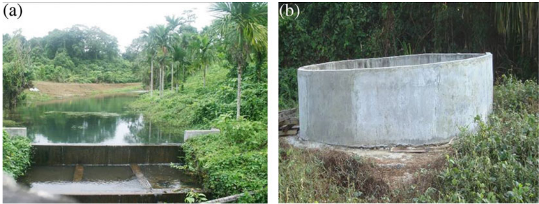
Fig. 7 Construction of (a) check dam and (b) well downstream of check dam (Garacharma farm, CIARI, Port Blair)
