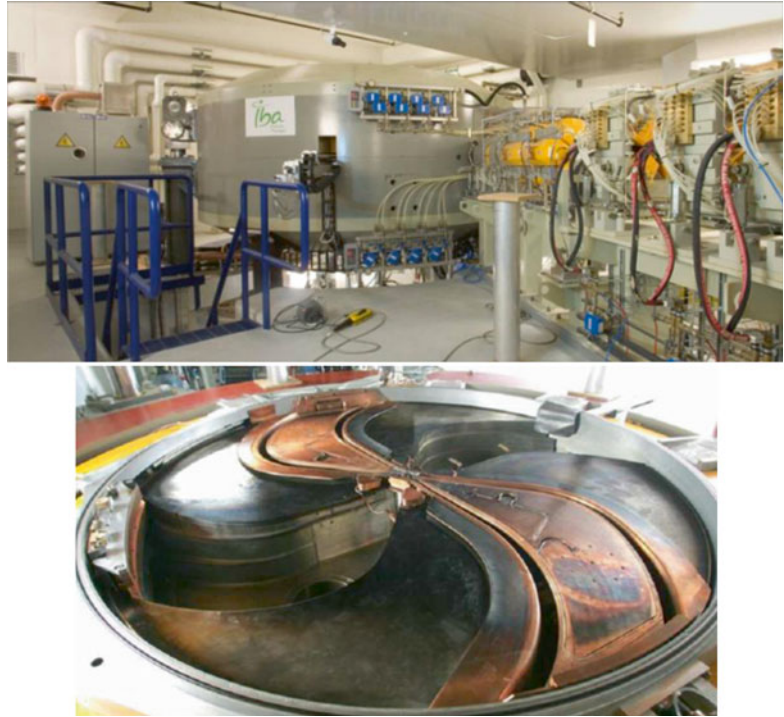
Fig. 3.10 External ( top image ) and internal ( bottom image ) view of the Cyclone®230 from IBA. The four sectors with spiraled poles and elliptical pole facing together with the two dees are visible
