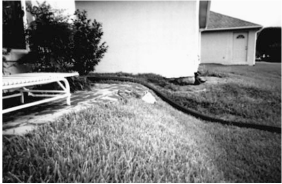
Fig. 33.3 View of subsided slope looking east
