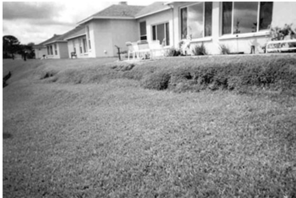
Fig. 33.2 View of subsided slope of adjoining house
