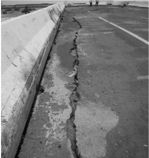
Fig. 30.4 Distress on the flexible pavement surface
