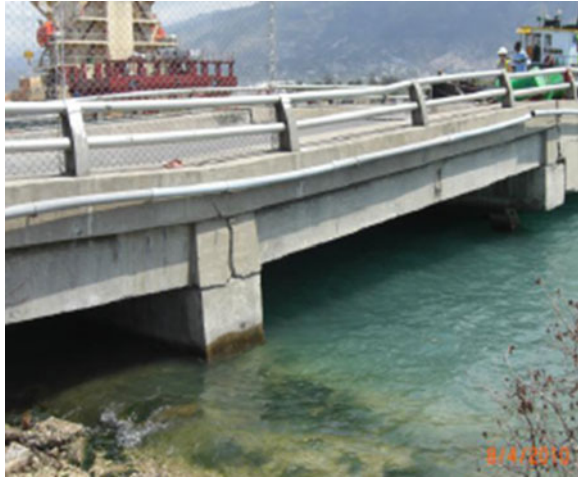
Fig. 28.13 Settlement of piers cause self-articulation of the bridge deck
