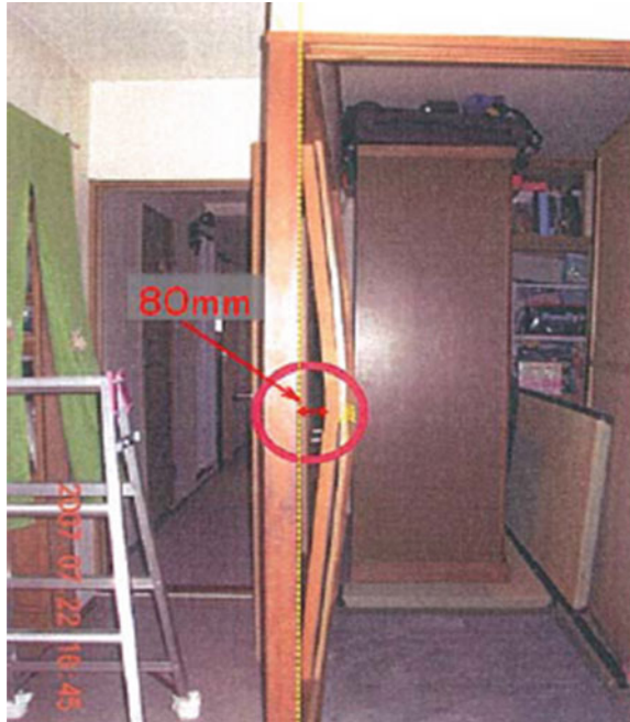
Photo 26.1 Buckling of a vertical door frame
