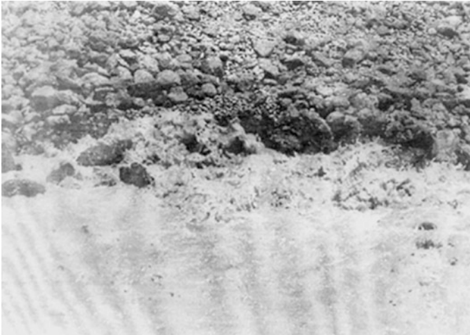
Fig. 21.2 The exit point of the leak as it appeared in the afternoon of August 16, 1984. Water surfaces under a substantial head and carry large quantities of suspended solids. The picture gives an idea of the grading of the latrine chunks used in the toe drain
