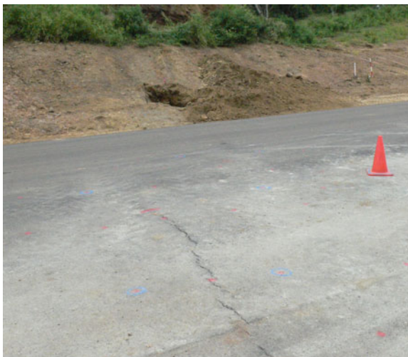
Photo 16.2 Shear movement in road pavement, Cut 3. February 2008
