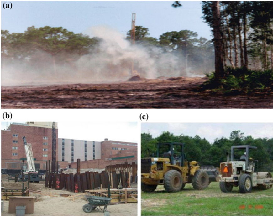
Fig. 34.1 Sources of construction vibrations. a Rock blasing at construction site. b Pile installation at hospital. c Vibratory compactor near surgical center
