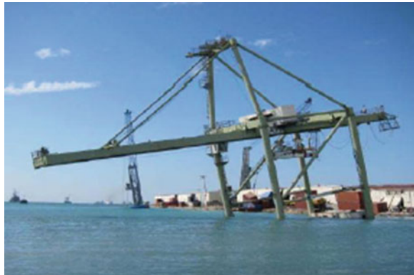
Fig. 28.9 Settlement of container crane in Port-au-Prince
