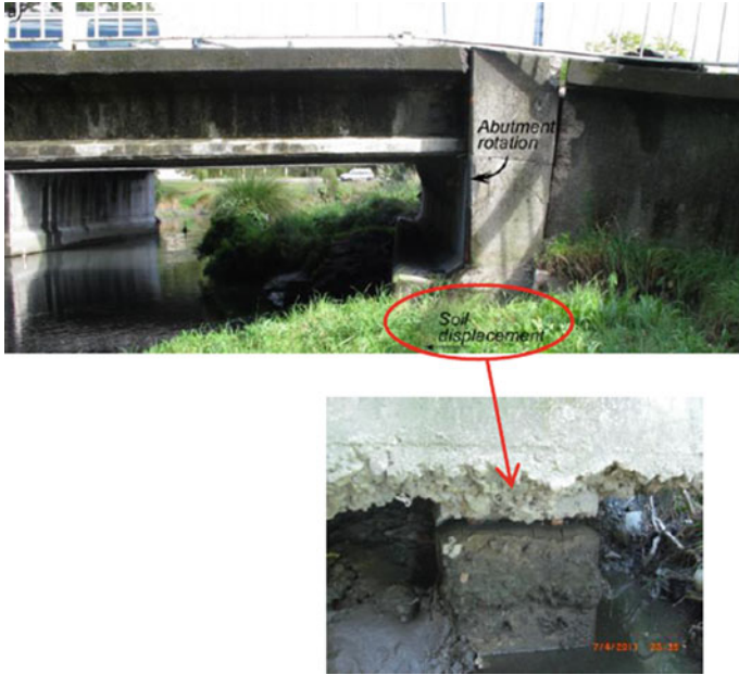
Fig. 28.6 Lateral spreading induced abutment rotation and shear failure of a square RC pile supporting the abutment
