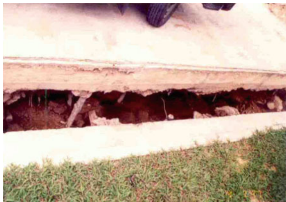
Fig. 18.1 Significant ground movement observed at an excavation site
