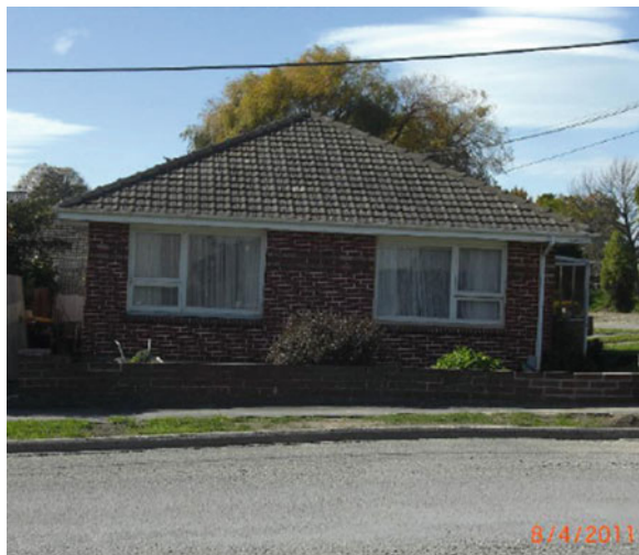
Fig. 28.3 Settlement/rotation of a residential building
