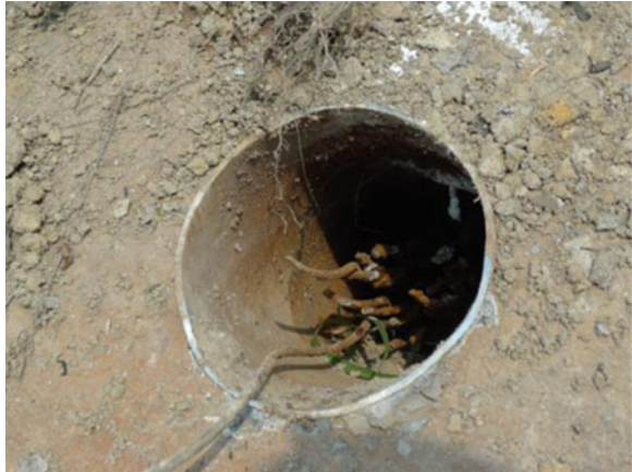
Fig. 15.9 Seriously corroded steel strands found from the back of a fallen anchor head
