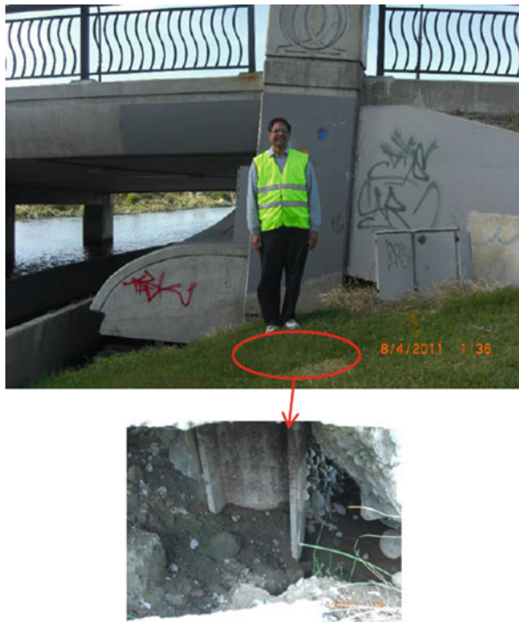
Fig. 28.7 Back rotation of a bridge abutment supported on steel H piles that formed plastic hinges at pile heads
