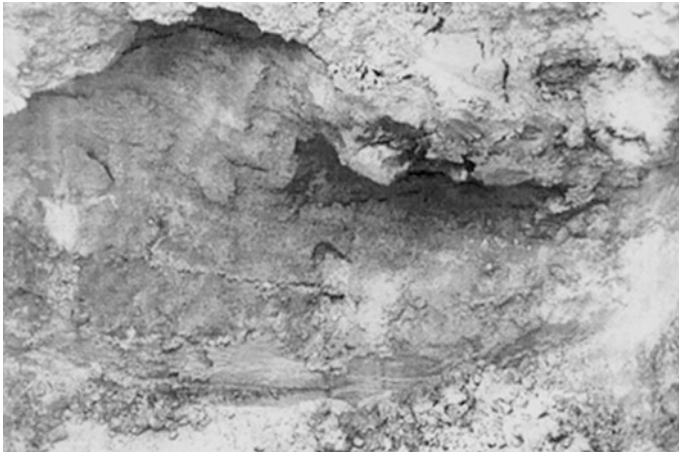
Fig. 21.3 The cavity across section 50 m u/s from the dam axis. The wine red material is the sand +gravel used to plug the leak. The cavity upper half is within the artificial clay blanket. The lower half of the cavity has been cut through the natural foundation
