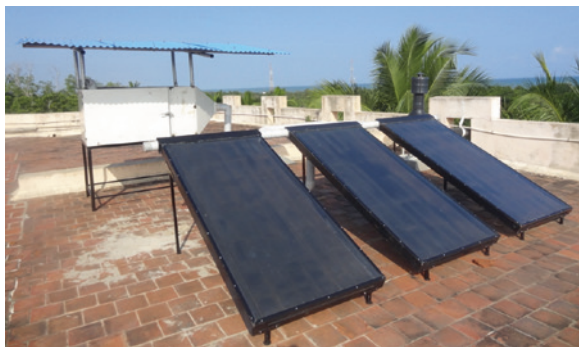
Fig. 5 Solar Dryer with wire mesh air heater—Pondicherry University
