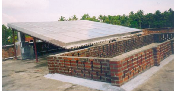
Fig. 4 Drier integrated with solar air heater—CUSAT
