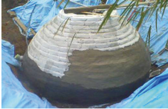
Fig. 10 Earth bag biogas plant (Geiger 2010)
