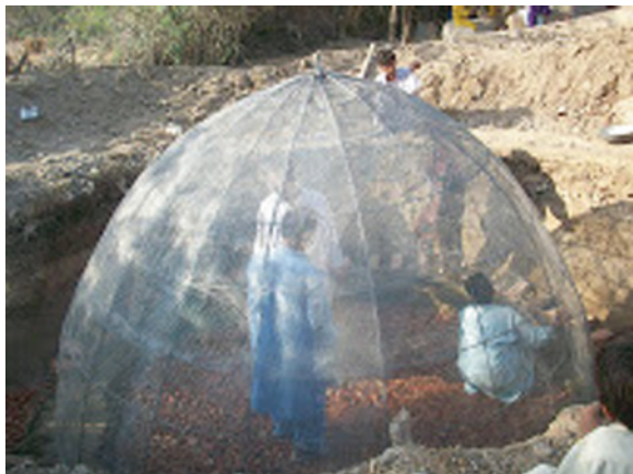
Fig. 11 Ferro-cement biogas plants (Construction of a biogas plant in Mirpurkhas Sindh Pakistan 2012)
