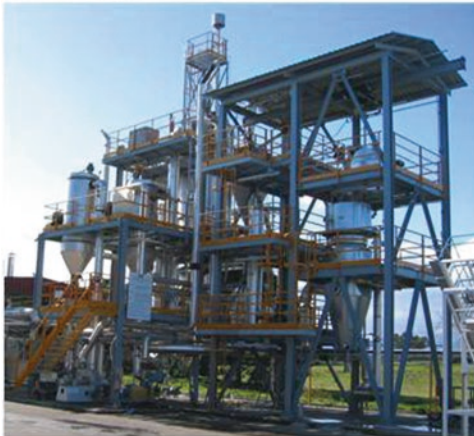
Internally circulating fluidised system comprises of a gasification zone fluidised with steam and a combustion zone fluidized with air.
