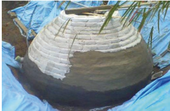
Fig. 10 Earth bag biogas plant (Geiger 2010)
