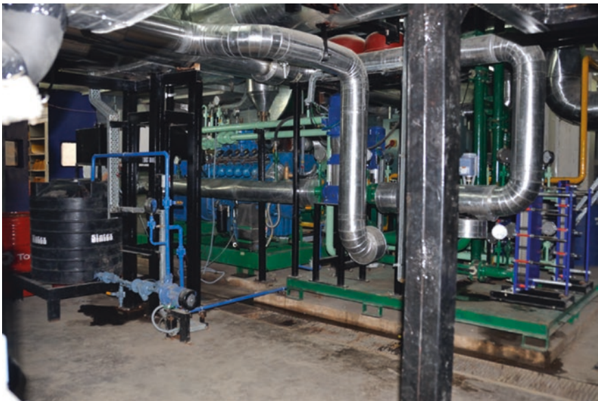
Fig. 6 An inside view of the Trigeration demonstration pilot plant at JPNATC
