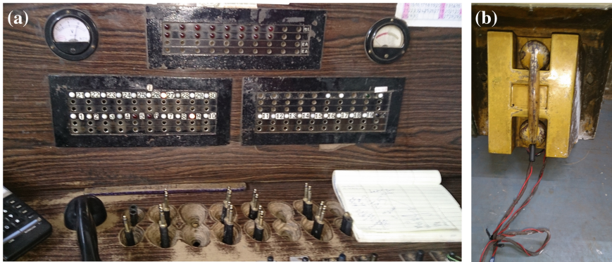
Fig. 3 Communication system at site C. a Chord based communication board at surface. b Telephone set
